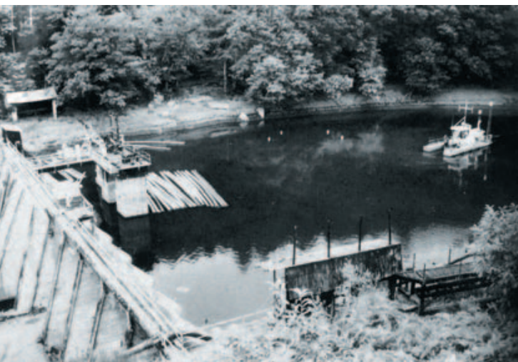
The Kernansquillec dam in 1996 during the pumping out of mud from the reservoir prior to drainage.
