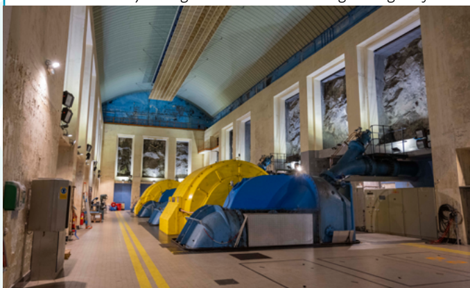
↑ Interior of the Montpezat powerplant
